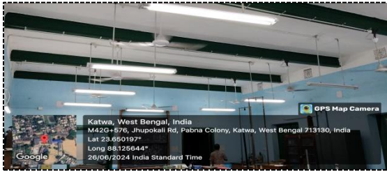
LED facility in the class room
